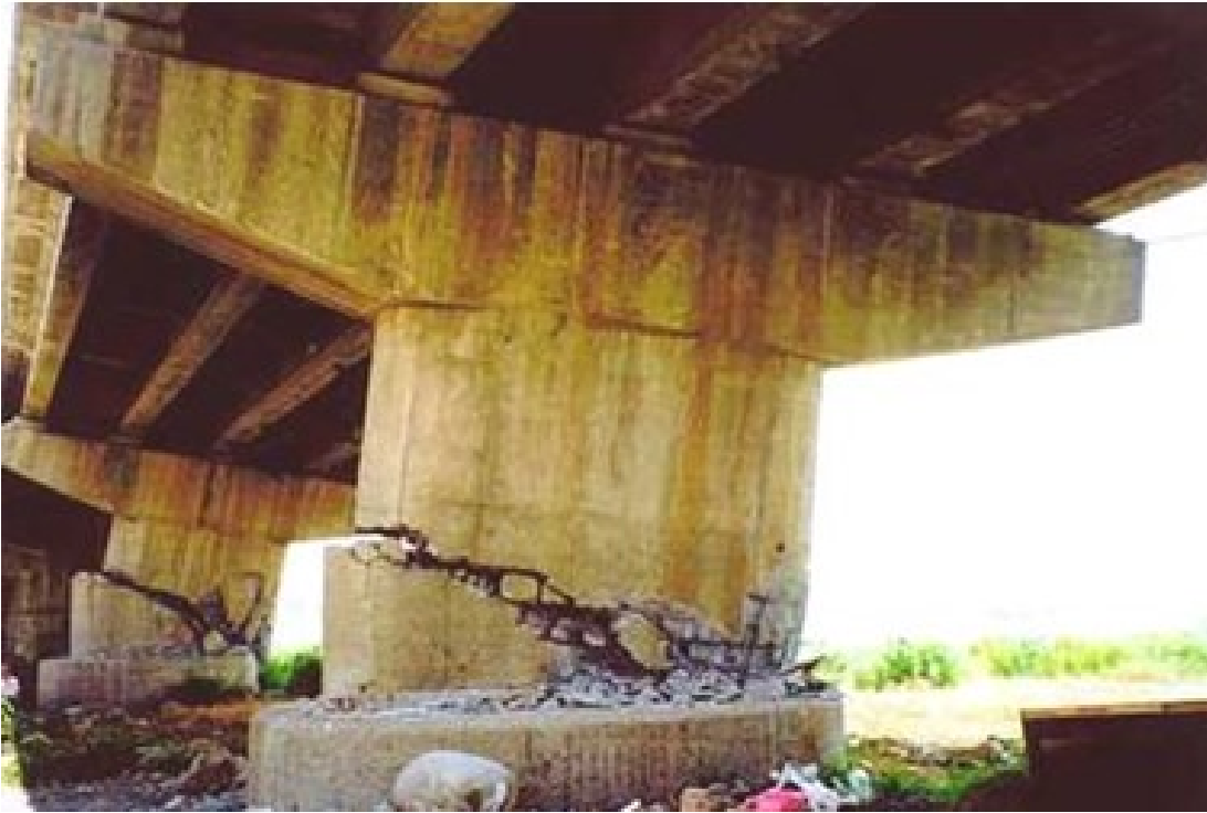
Figure 9. Tilting and failure of the piers of Wu Creek Bridge during the 921 Jiji Earthquake (National Center for Research on Earthquake Engineering, 2020).
