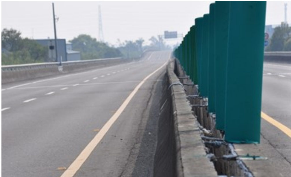
Figure 7. The uneven opening depicted in Figure 6, which leads to road surface bending on the left.
