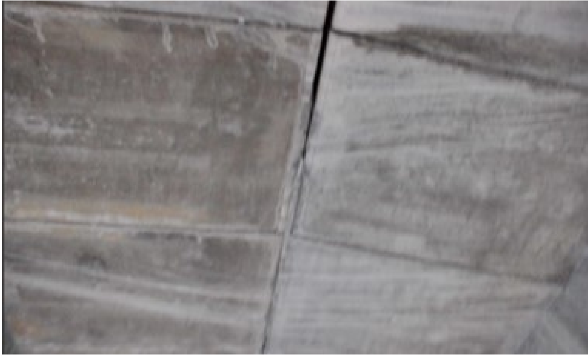
Figure 5. Fracture of the box girders on two adjacent land bridges without seismic isolation pads, resulting from excessive mutual compression.
