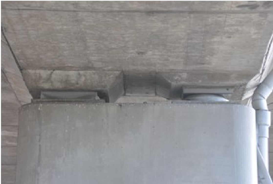
Figure 3. Seismic isolation pad positioned between the bridge pier and the box girder.
