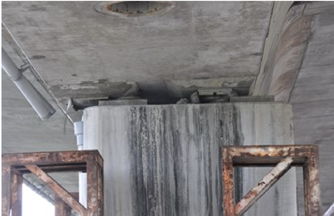
Figure 8. Shear failure of the isolation pad, causing the bridge deck to shift 55 cm to the left relative to the bridge piers.
